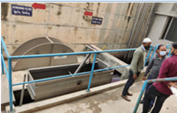
Mechanical screen and lifting tank
