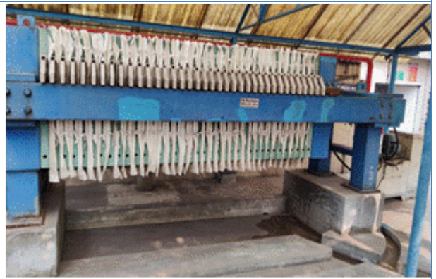
Sludge dewatering filter press
