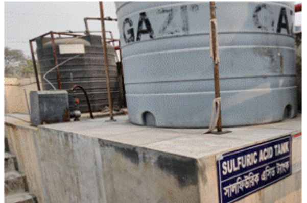
Chemical dosing system
