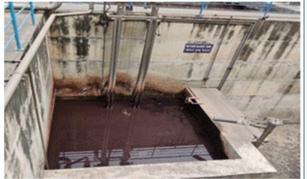
Sludge recirculation tank
