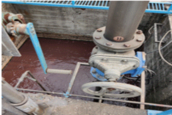
Sludge recirculation tank
