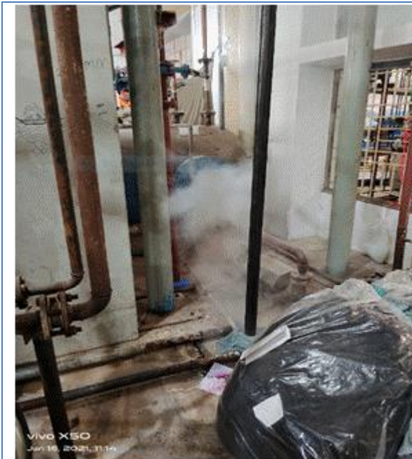
Steam leakage in dyeing
