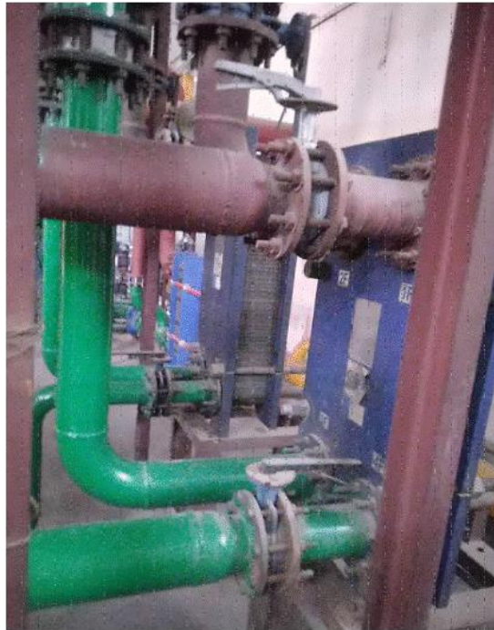
Figure 12: Jacket water cooling PHE
