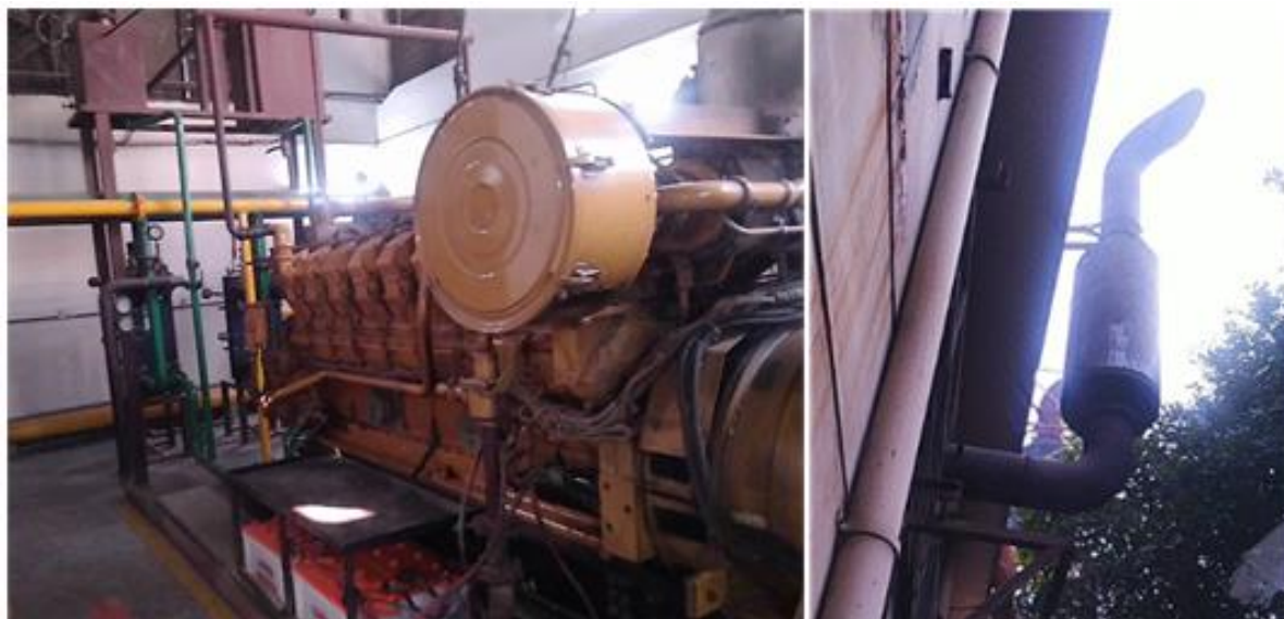
Figure 9: Gas Engine exhaust gas duct
