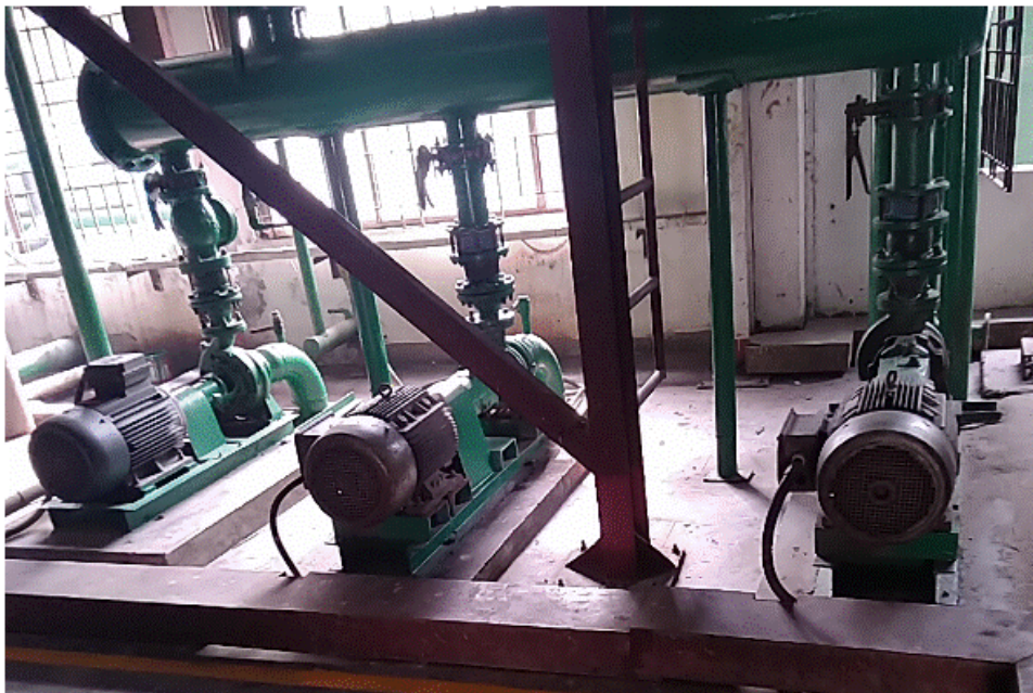
Figure 20: WTP Service Pumps
