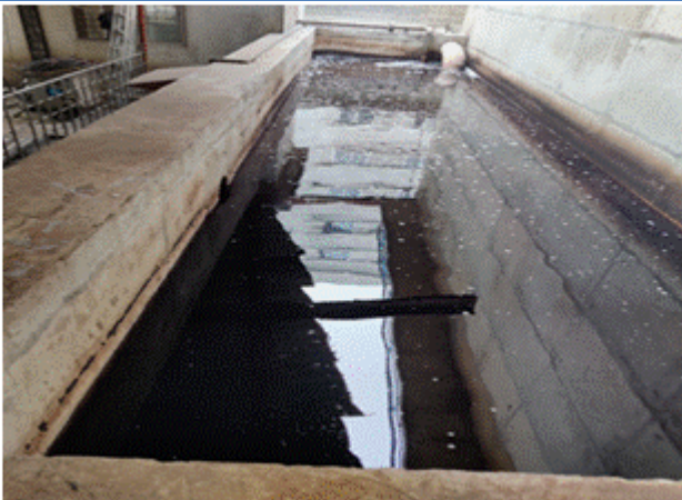
Post aeration tank
