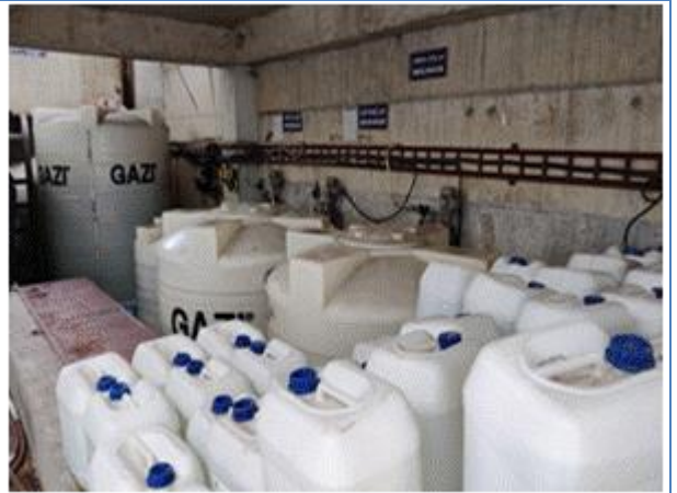
Chemical dosing system
