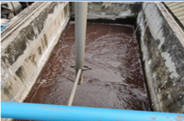
Sludge holding tank
