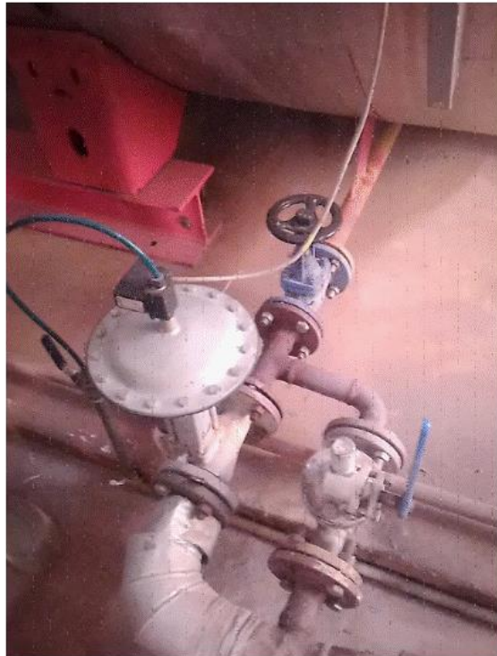
Figure 15: Manual blowdown practice
