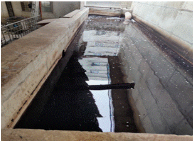
Post aeration tank
