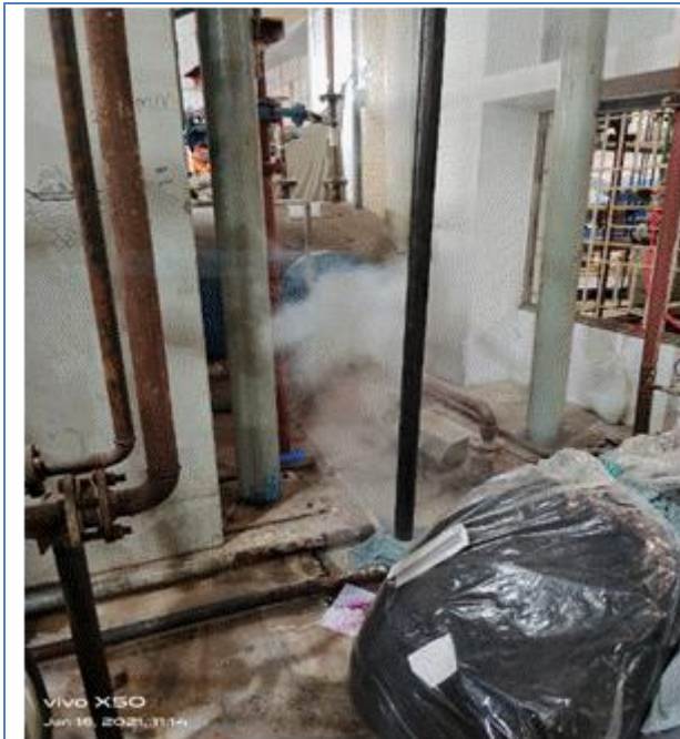
Steam leakage in dyeing
