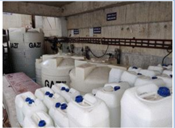
Chemical dosing system
