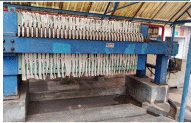
Sludge dewatering filter press
