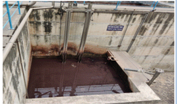
Sludge recirculation tank
