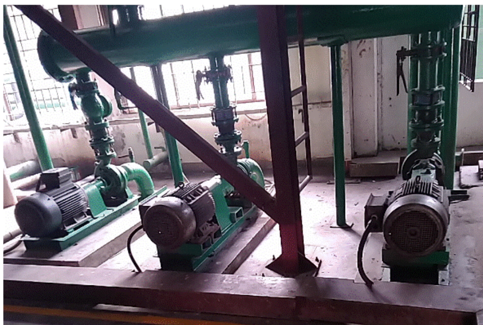
Figure 20: WTP Service Pumps
