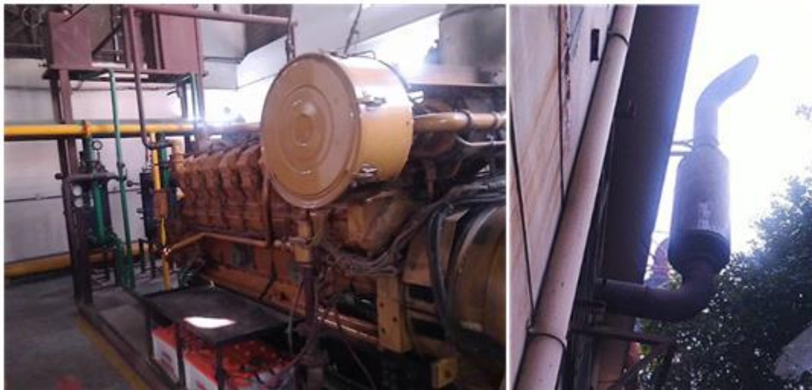
Figure 9: Gas Engine exhaust gas duct
