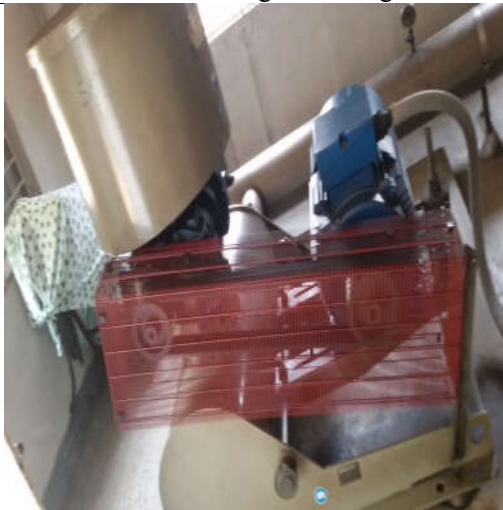
Secured rotating parts in ETP blower room
