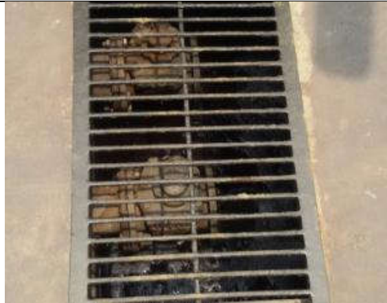
ETP discharge point
